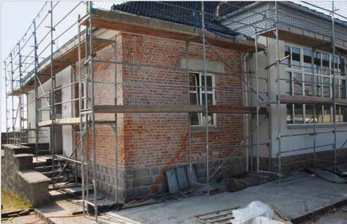
Façade of the former infirmary building in scaffolding during renovations; the building is being used as a museum. The section of the building without plastering functions as a 'historical window' onto how it looked in 1945 (© Federal Ministry of the Interior/Stephan Matyus).
