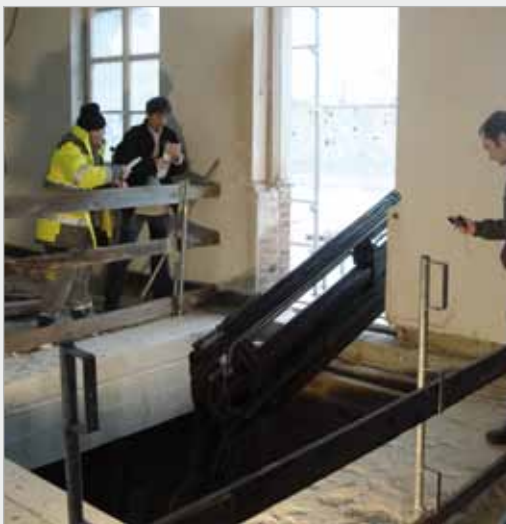
Photograph of construction work to install a lift that will make the building accessible to people with impaired mobility (© Federal Ministry of the Interior/Robert Vorberg).
